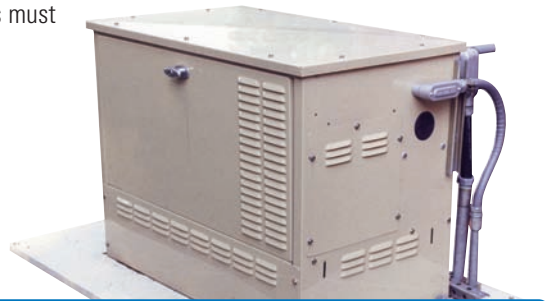
Typical stationary natural-gas fired generator
