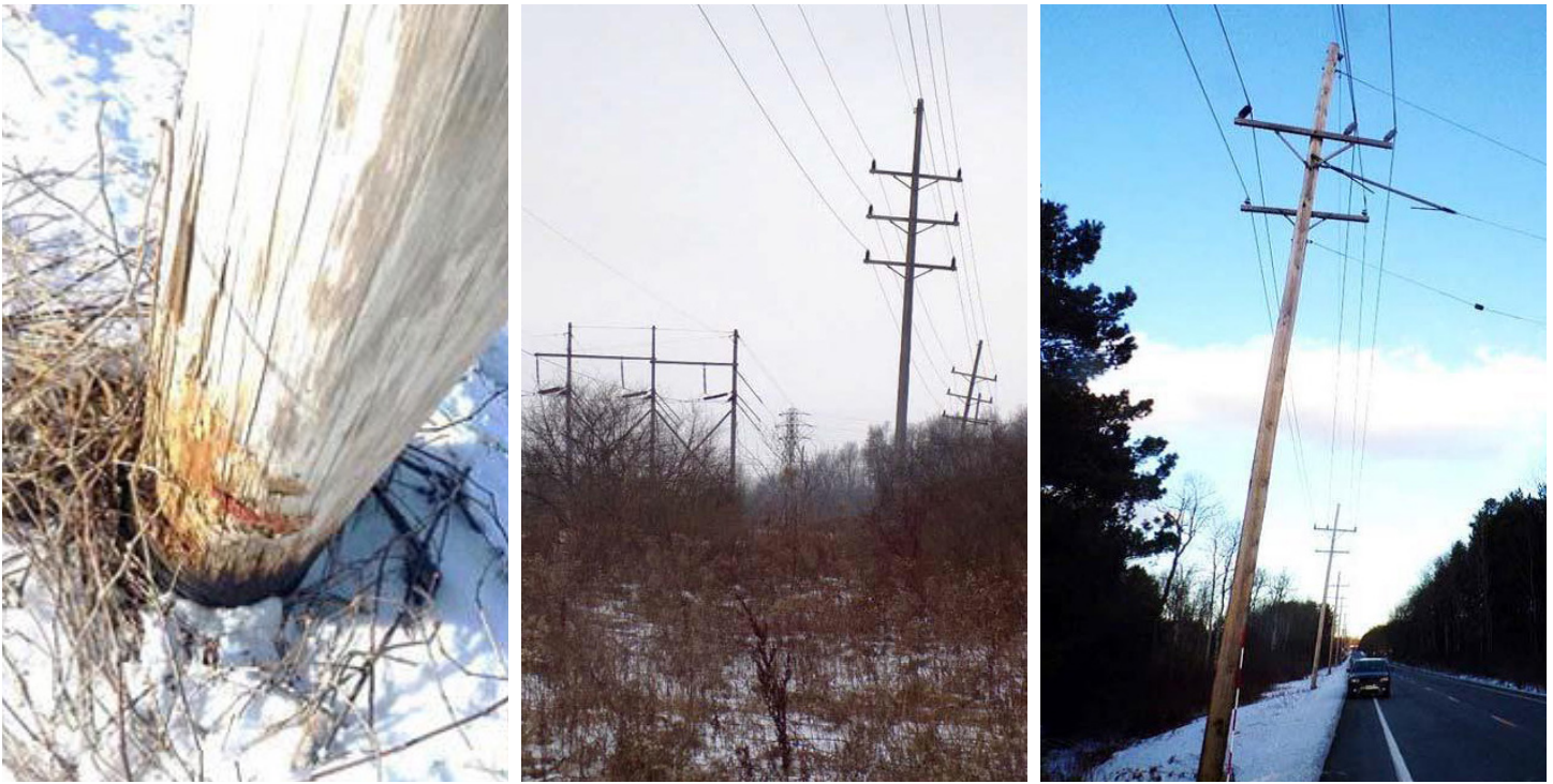
Field assessments and structural analysis conducted in February 2019 in support of the rebuild project
