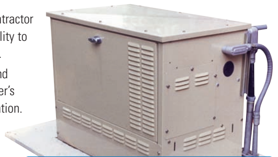
Typical stationary natural-gas fired generator
